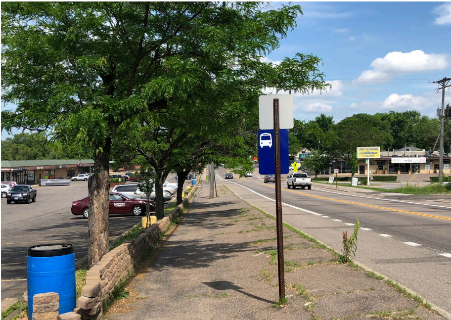
Photo of asphalt walkway along Minnetonka Blvd that needs maintenance and updating to be more welcoming
