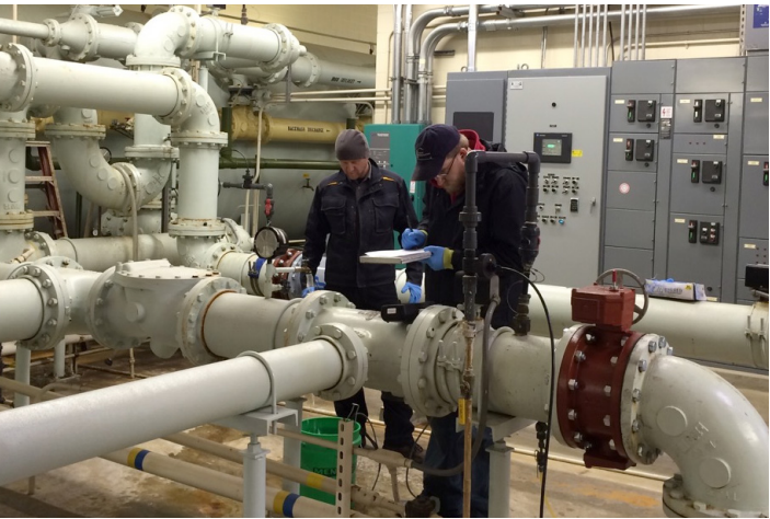
Drinking water treatment plant.
